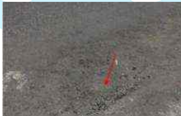
Gambar 2. 17 Pelepasan Butir ( Weathering/Raveling )
